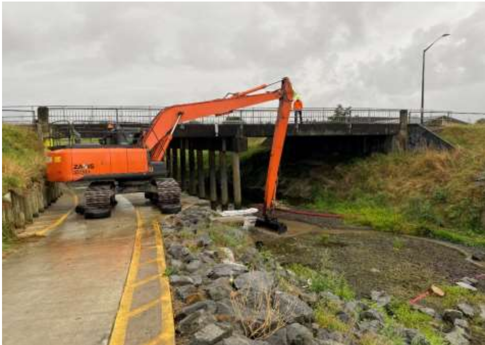
Figure 3 Long reach digger removing rooted alligator weed plants in gravel beach. (K.Hoggard)
